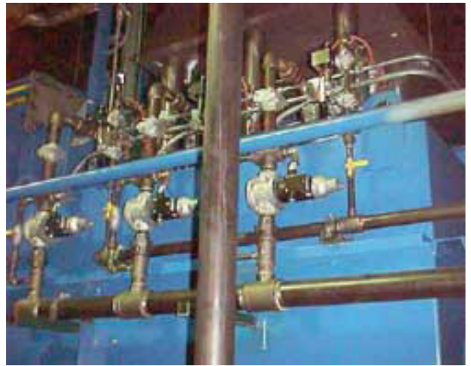
Six Kromschroder BICR single-ended, self-recuperating burners, a flame-management system, and Kanthal APM radiant tubes reduced gross heat input to the furnace by 22%.
