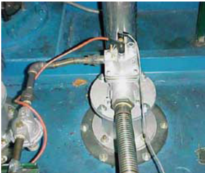
Kromschroder flame-management system, combined with other upgrades, reduced furnace fuel consumption by 40%.
