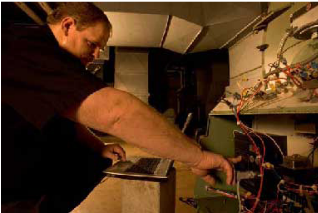
Butch Harvey checks the status history of the BCU 370 installed at Lincoln High School. Flame strength, configurations parameters, and error history can all be viewed via the included 2 digit display. Complete control history and trending can be obtained using Kromschroder's BCSoft PC software.
